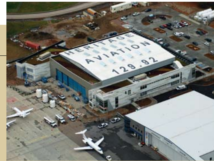
An aerial view of the almost complete Heritage Aviation Hangar and Office Building.
